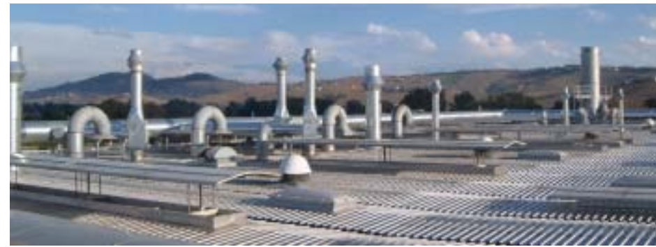
Plant section showing the ducts for capture of polluted air originated by the wet-paint booths
