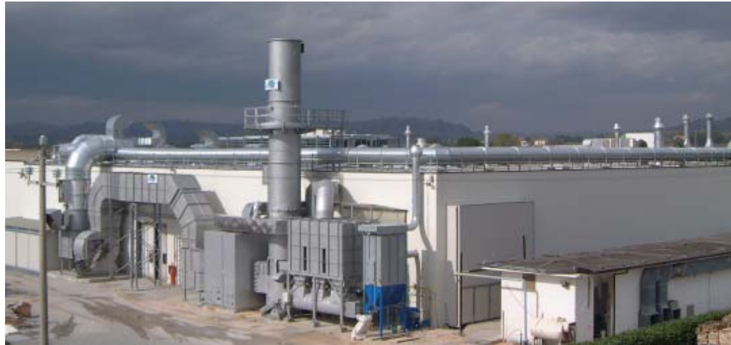
Overall view of the solvent abatement plant
