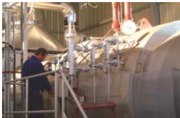
The picture above gives an idea of the impressive size of the post-combustion unit, and not surprisingly since it is the largest of its kind installed in Europe, with a nominal capacity of 250,000 Nm 3 /h, increasable to 275,000 Nm 3 /h. It allows also the production of 12 tonnes per hour of steam at 9 bar using the solvents' enthalpic energy and manages 38 ink laying machines, handling them independently from each other.
