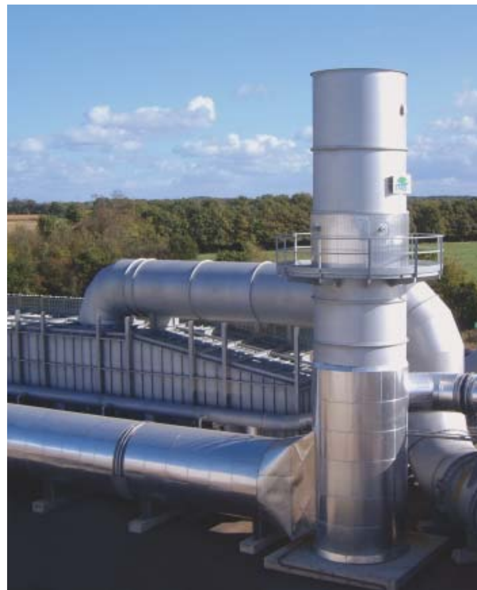
View of the Rigetherm® post-combustion unit (with the steam boiler's recovery system), soundproofed cabin, control station and process fan.
